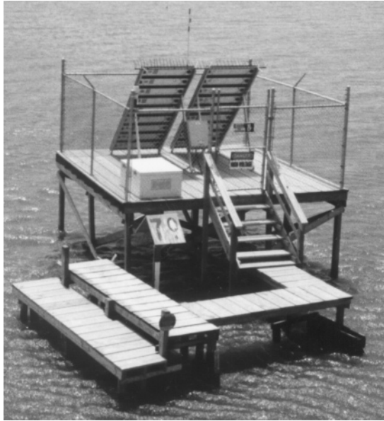
Figure 10.6 Typical solar electric CP installation. (Courtesy of Kyocera Solar, Inc.)
